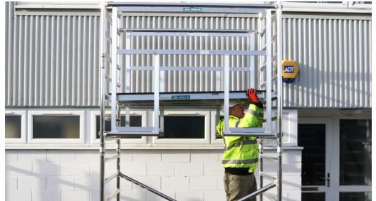
10. Fit 1 trap and 1 plain platform to the 3rd rung down. Making sure the trapdoor is with the ladder section.
