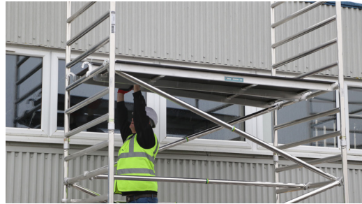
16. Fit your working platforms on the 6th rung down from the top of the tower ensuring the trap is opening outwards to the tower and inlin with the trap platform below. If needed, reposition your temporary board from below.
