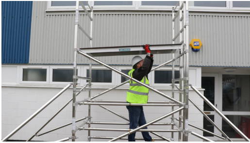
13. Fit trapdoor platform on ladder side 3rd rung down from the top.
