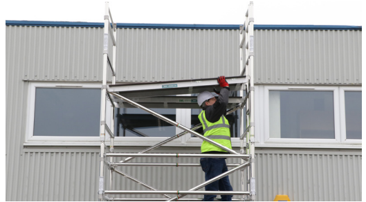
16. Fit your working platforms on the 3rd rung down from the top of the tower ensuring the trap is on the ladder side opening outwards. If needed, reposition your temporary board from below.
