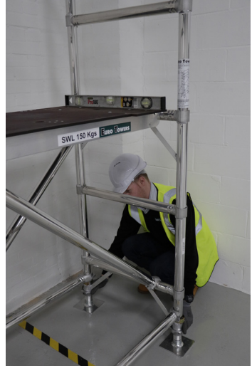
6. Level the tower adjusting the leg nut using a spirit level as a guide.
