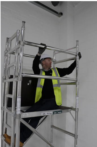
7. Sitting through the trapdoor fit 4 horizontal braces to the verticals above each rung of the frames above the platform to complete a guardrail.
